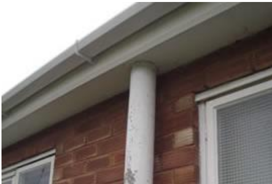
Asbestos cement drainage pipe (downpipe)
