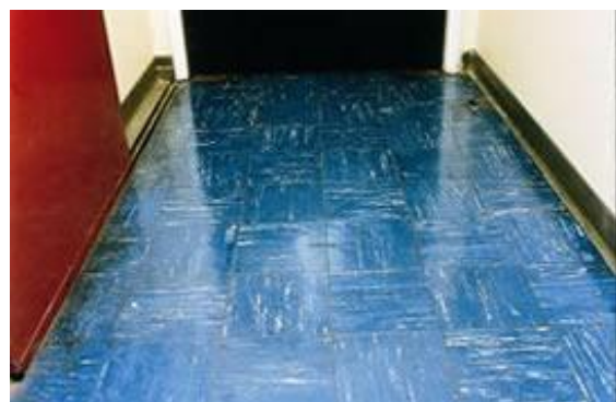
Asbestos containing floor tiles in a corridor
