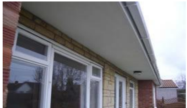
Pieces of Asbestos Insulating Board (AIB)
