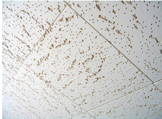
Asbestos containing ceiling tiles
