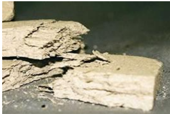
Pieces of Asbestos Insulating Board (AIB)
