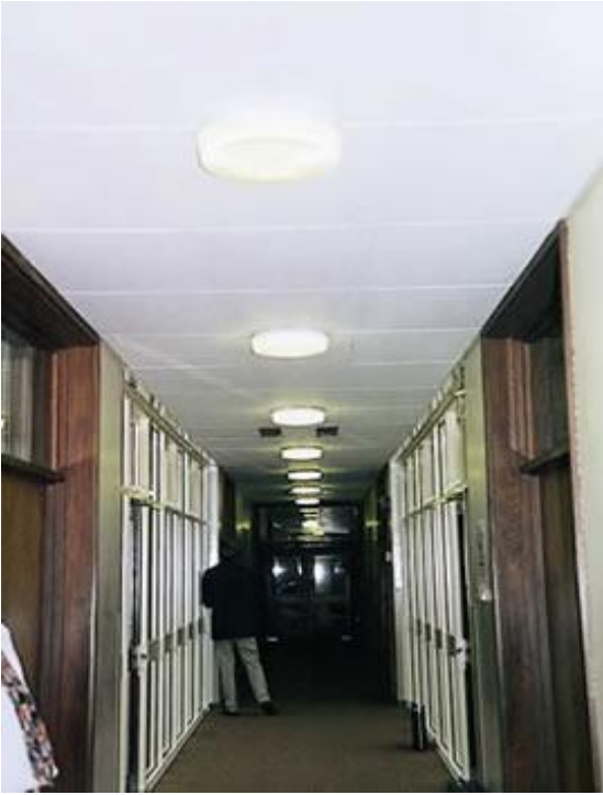
Suspended Asbestos Insulating Board tiles in a corridor
