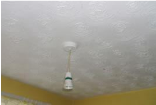
Asbestos textured coating
