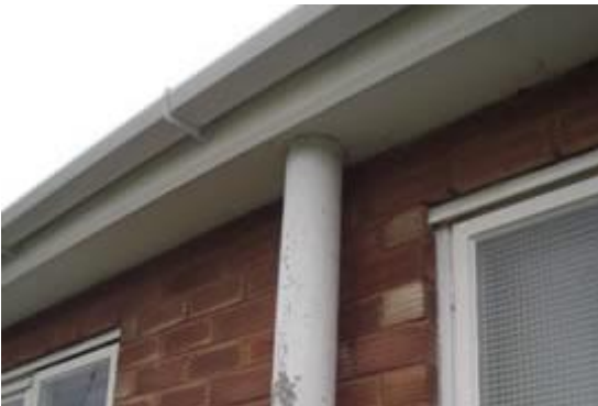
Asbestos cement drainage pipe (downpipe)
