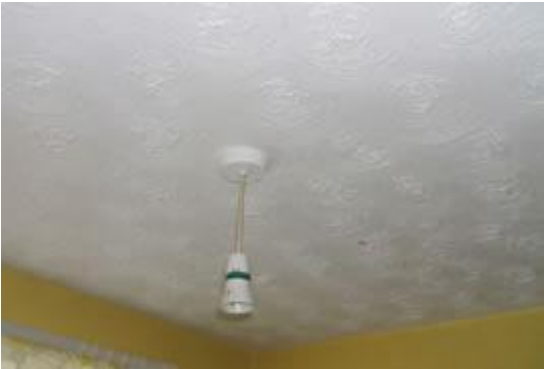
Asbestos textured coating
