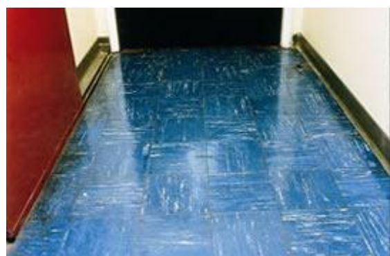
Asbestos containing floor tiles in a corridor
