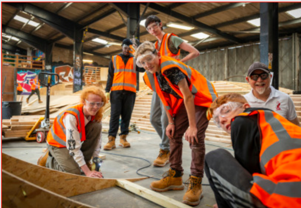
Pictured: one of our first projects in the Nottingham area, building Flo Skatepark.
